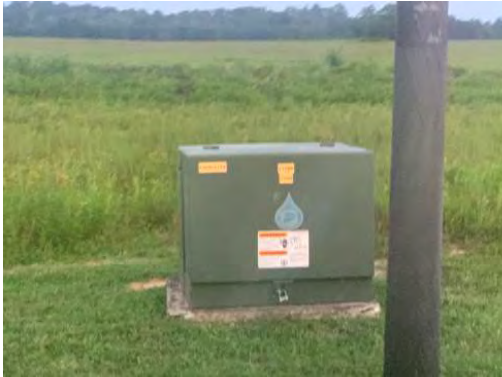
Property Photograph 3 – Pad-mounted electrical transformer on Property
